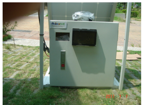
▲ DC/AC Control Box
