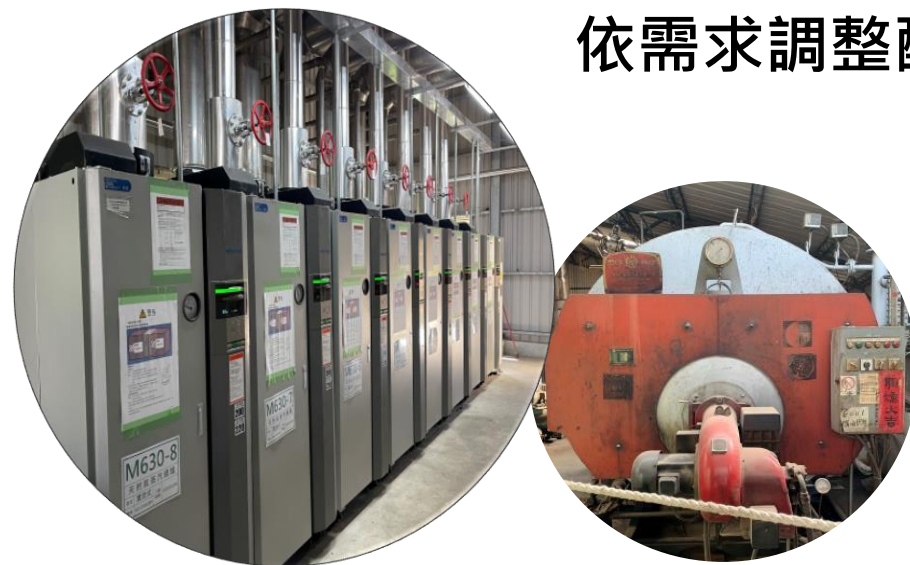
串聯燃氣鍋爐+備用燃油鍋爐
